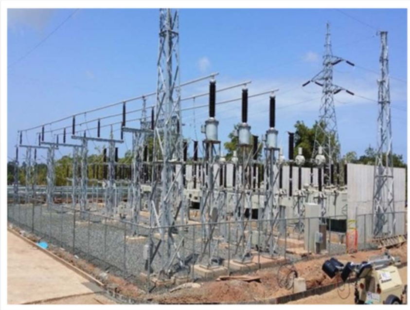
115kV Substation for JINRO Power 57.8MW PPS
