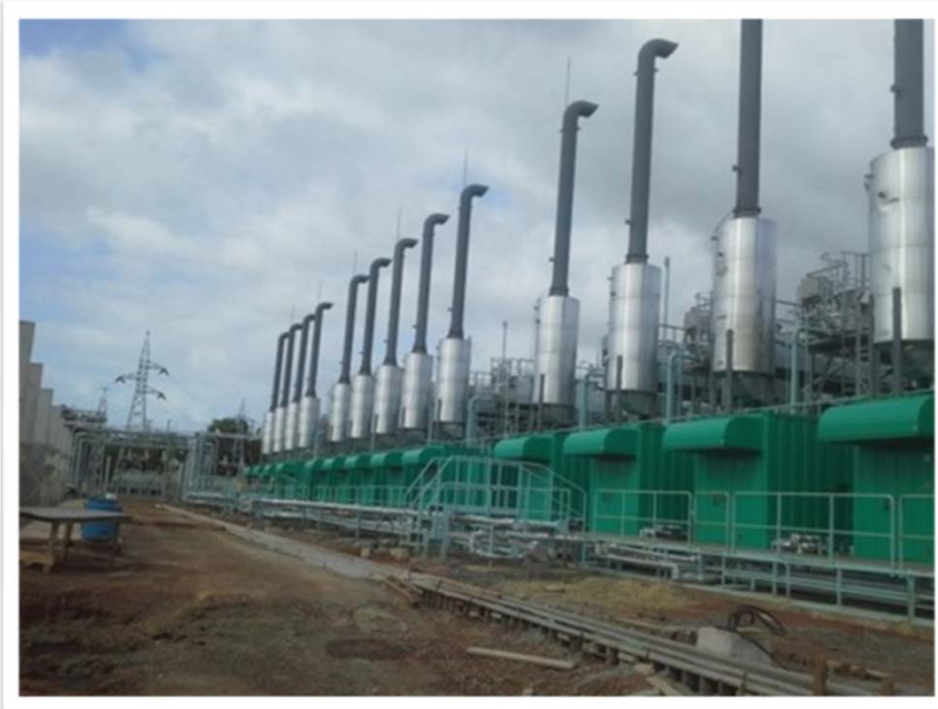
JINRO Power 57.8MW PPS
