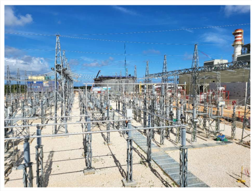
115kV Substation for Ukudu 198 MW CCPP
