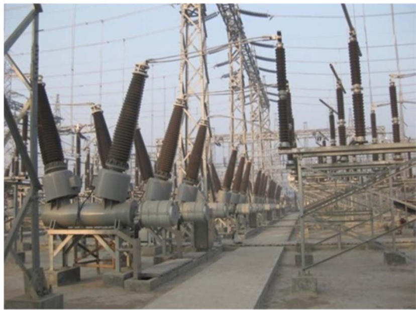
Fabrication of 230kV Gas Circuit Breaker(Jan.30, 2013)
