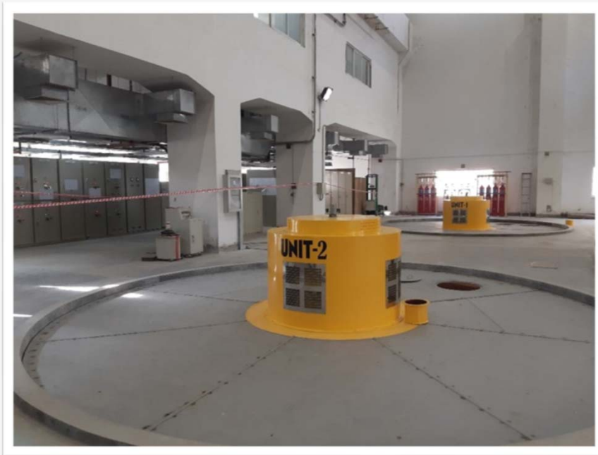
Hydro Power Generator
